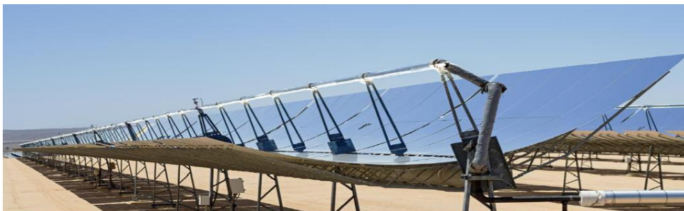
Fig. 1. Solar installation based on double-sided photomodules and a two-axis tracker
